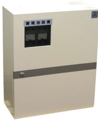
Storage battery equipment for emergency lighting (2) L48R7D-N
